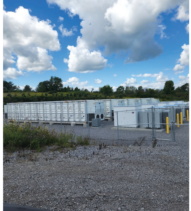
Orangeville Energy Storage, LLC, AC battery energy storage facility
